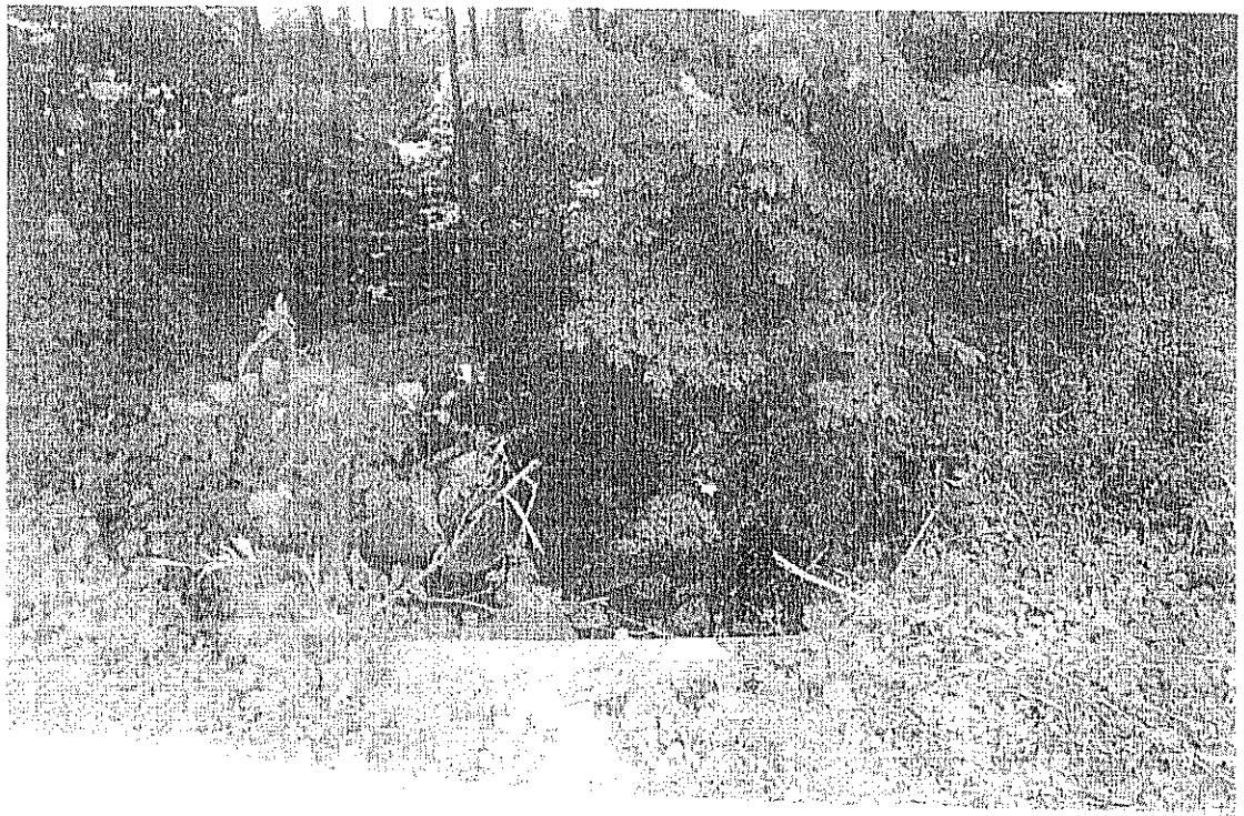
Picture P7 – Looking upstream from the u/s face of existing Rt. 202 culvert Picture Taken: 11/29/2007
